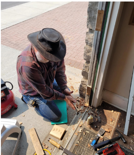
Guy Davis repaired, refitted and restrained St. Margaret's Cody St. and Montreal Rd. doors in 2025—the main "Maintenance, Repairs" expense noted above. His work was exceptional— and he brought his own kneeler.
